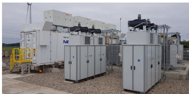
Figuur 4.1 GIGA Rhino battery container on site
